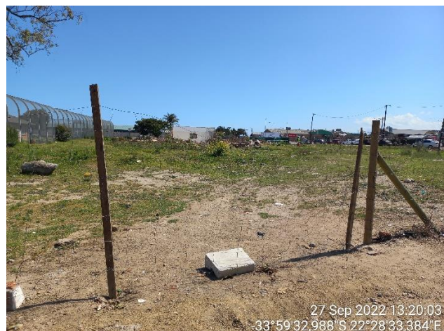
Figure 5: View west at site entry/exit point off Golf Street. Note partially demolished building in centre of site.
