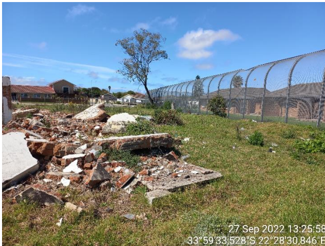
Fig.19: Rubble remaining of site from old building.
