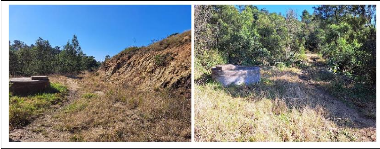
Figure 3. Example of the bulk sewer line installed on the opposite side of the Skaapkop River in Pacaltsdorp where the sewer line has become a single lane dirt track following benching. Photo credits: J. Dabrowski.
