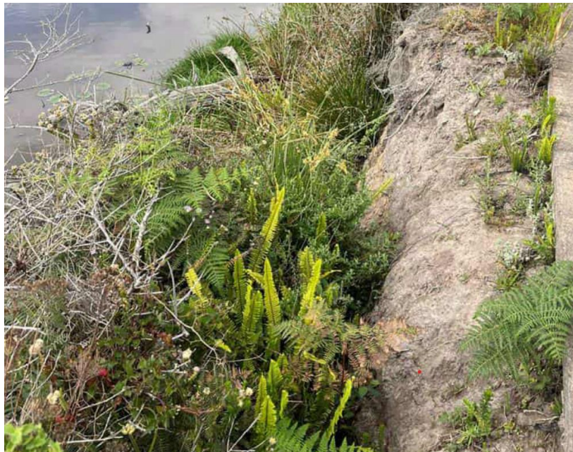
Figure 2. Image of eroding dam wall along the walkway (SMEC, 2023).
