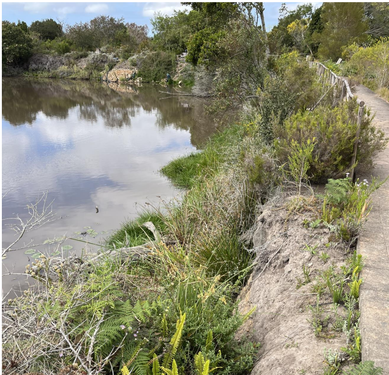
Figure 4-2: Existing eroded embankment
