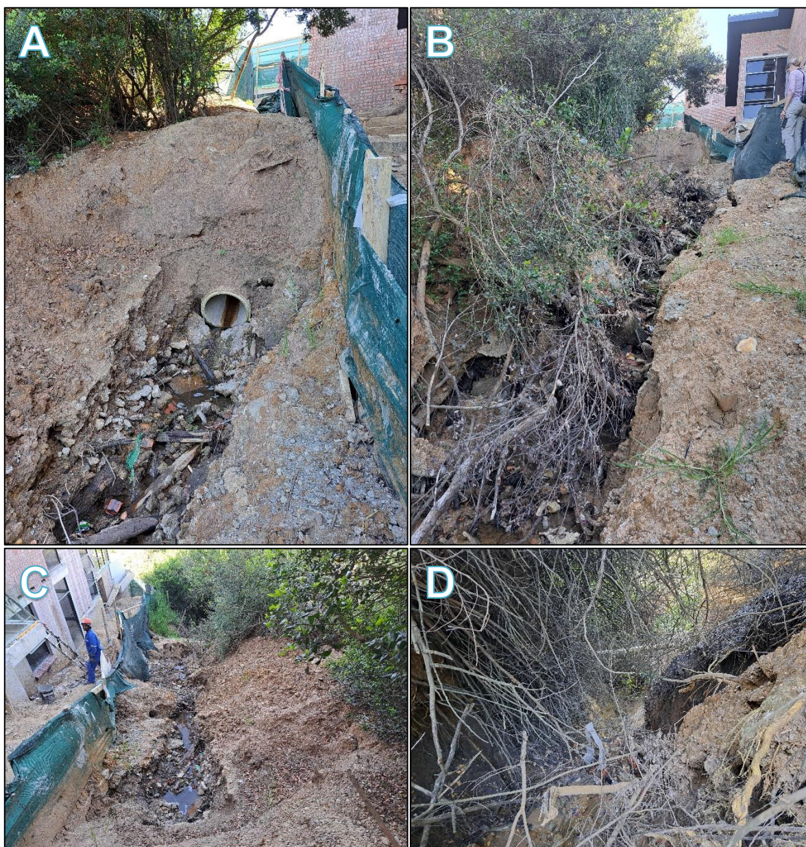
Figure 5: Photographs of the eroded channel below Voëlklip Road including the stormwater outlet discharging into the channel (A); a view of the eroded channel to the north (B); view of the eroded channel to the south (C); and the heavily eroded banks of the channel (with the sewer pipe crossing in the background (D)).
