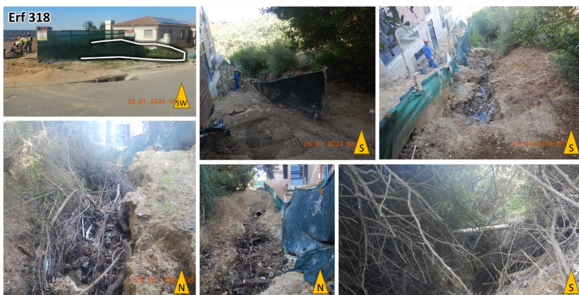
Figure 9: Photos of the site taken on Erf 318. This site is being eroded, and a large house is being constructed east of the erosion on the site.
