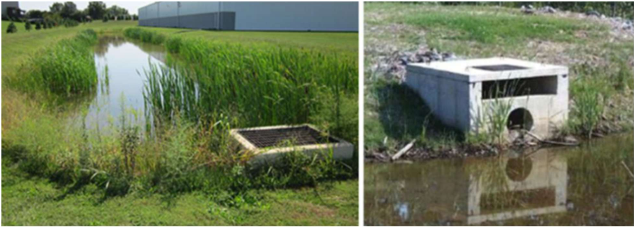
Figure 2-3 Ponds and Overflow Inlet Structures
