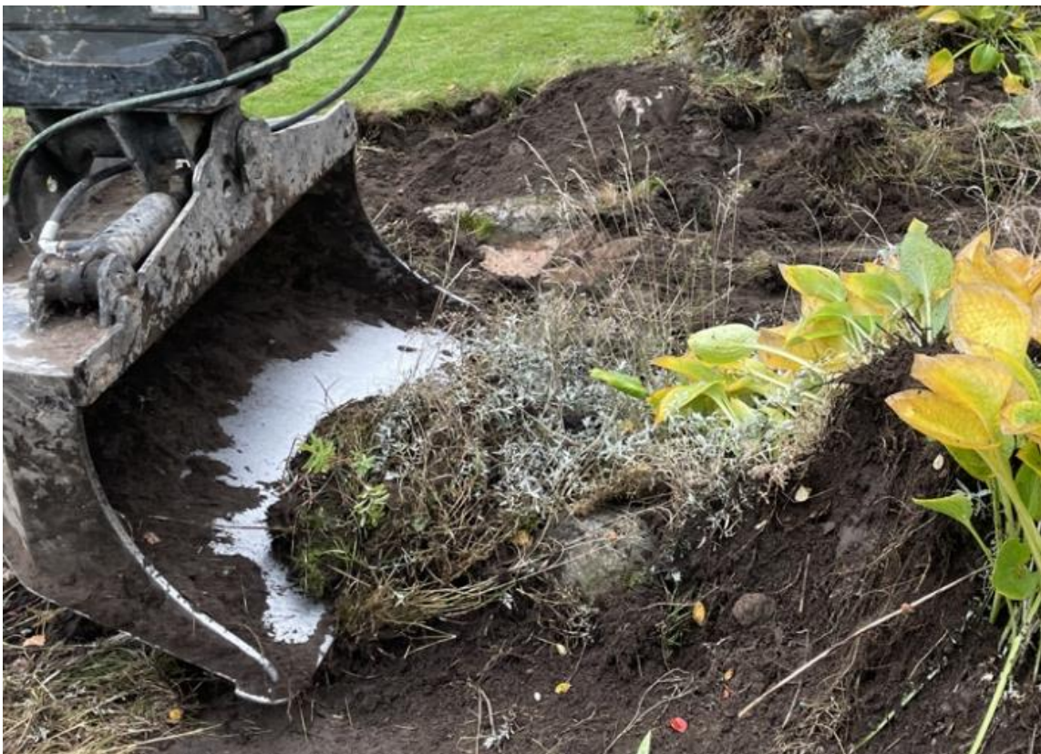
Figure 17: An example of an excavator carefully lifting plants in order to minimise soil disturbance.
