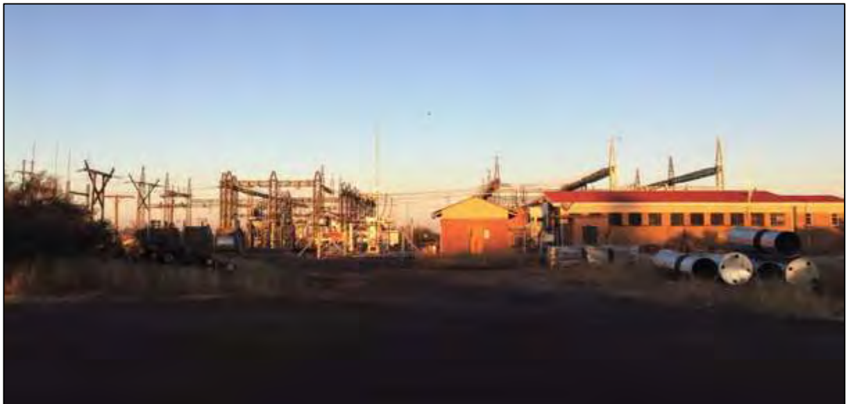
Figure 22: View west from Photo 6 of the existing Hotazel Substation to which the proposed power line would be routed.
