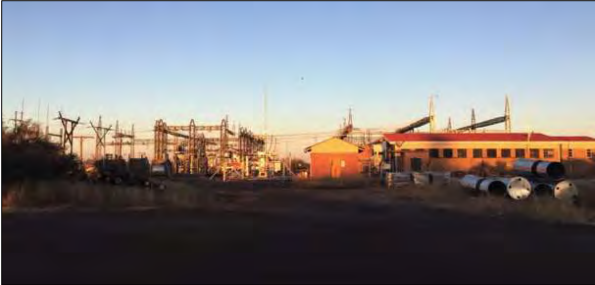
Figure 51: View west from Photo 6 of the existing Hotazel Substation to which the proposed power line would be routed.
