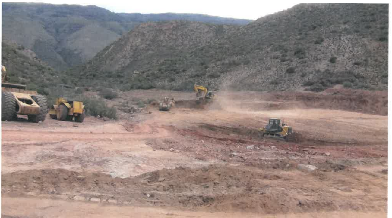
Photo 2: View (taken from the newly constructed dam wall) of the construction of the new dam within a watercourse with associated vegetation clearing and excavation of soil evidently taking place on the property.
