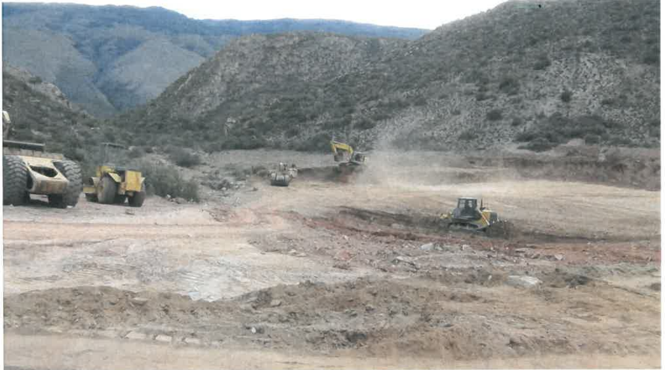
Photo 2: View (taken from the newly constructed dam wall) of the construction of the new dam within a watercourse with associated vegetation clearing and excavation of soil evidently taking place on the property.
