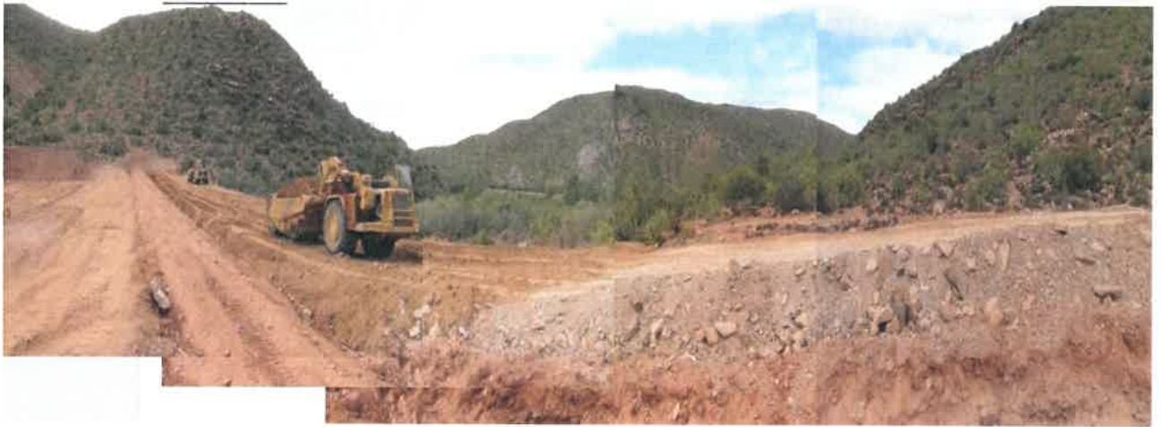
Photo 1: View of the construction of a new dam wall within a watercourse on the property.
