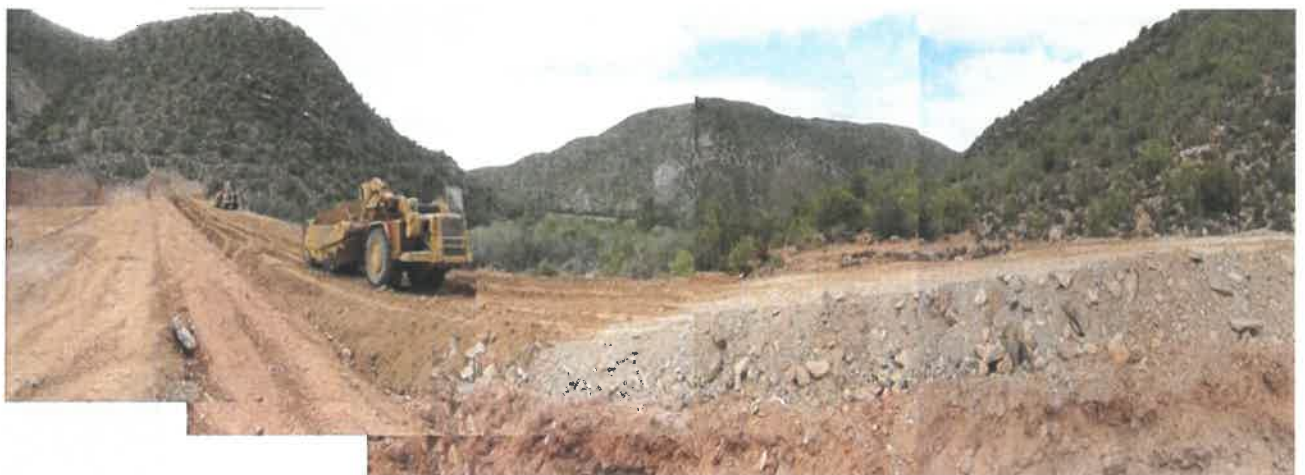
Photo 1: View of the construction of a new dam wall within a watercourse on the property.
