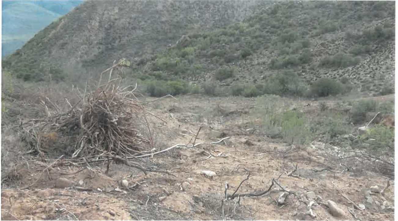
Photo 3: View of the destruction of vegetation cleared and topsoil disturbance within a watercourse with the construction of the new dam on the property.
