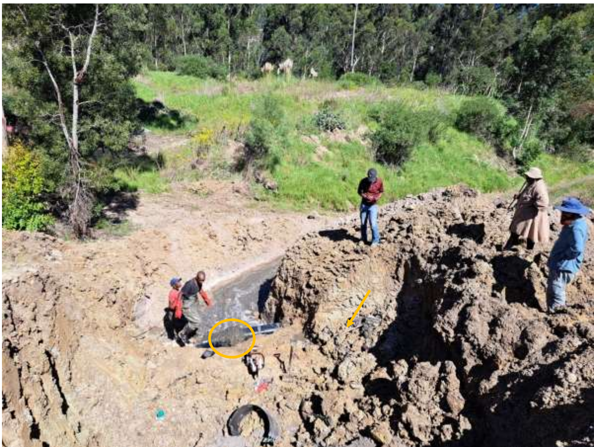
Figure 10. Photo taken on 31 March 2023 of a bulk sewerline that was opened to remove a blockage due to a walking crutch (arrow). Raw sewage and silt flowed straight downslope into the Bigai Wetland.
