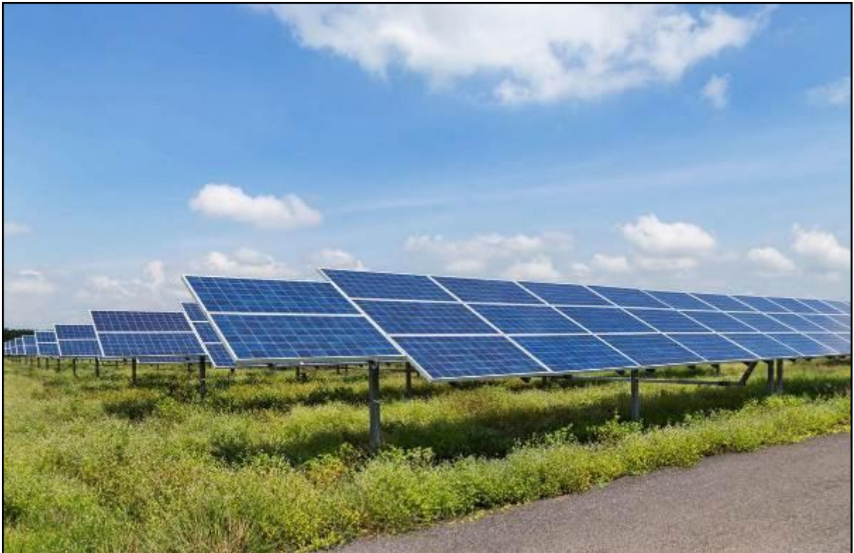
Photograph 1.1: Typical PV SEF facility
