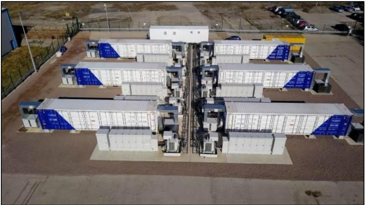
Photograph 1.2: Example of BESS located in storage containers
