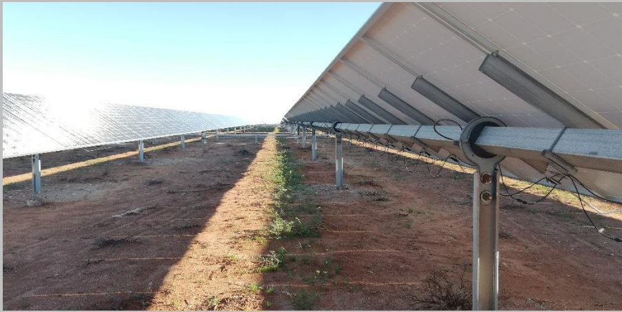
Figure 9: Showing vegetation re-establishing along the driplines of the arrays within weeks after installation.
