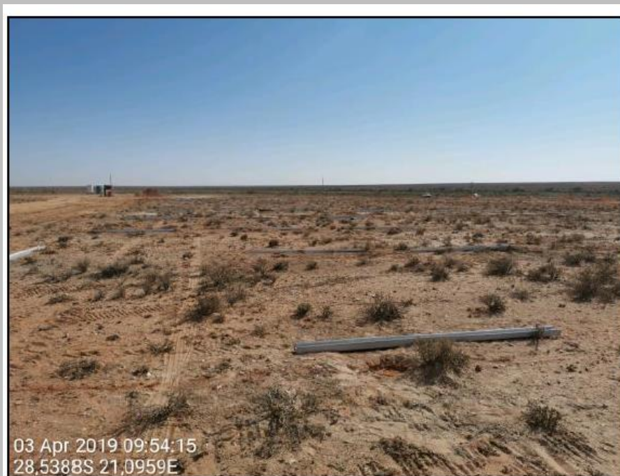
Figure 6: pre-drilled holes are backfilled with a wet sand mixture and steel piles placed in position ready for ramming.
