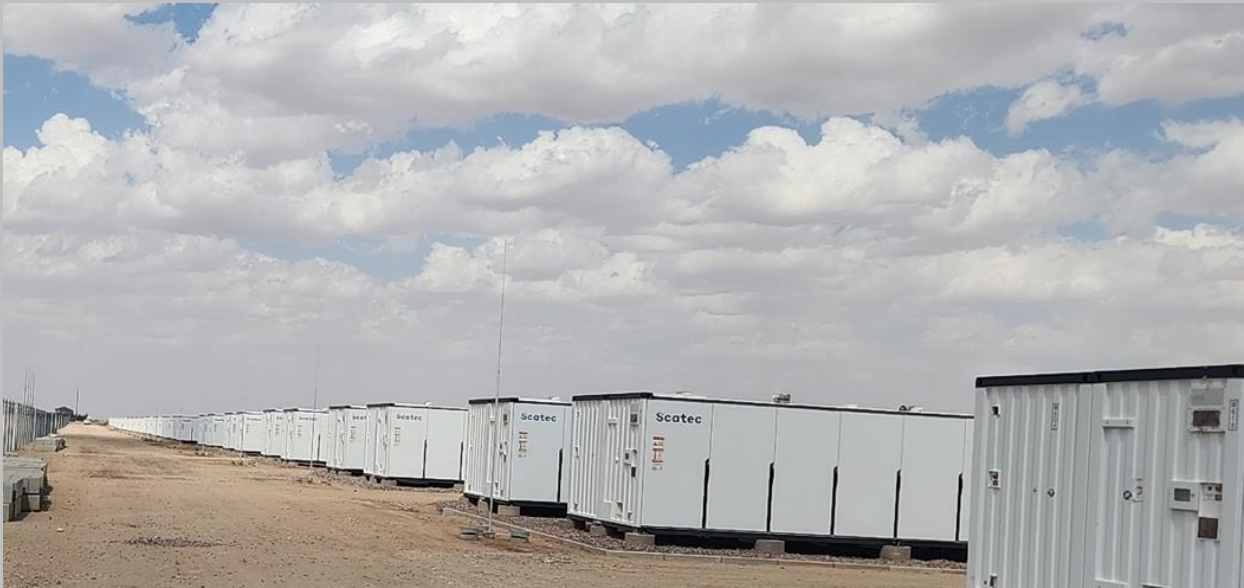
Figure 11: Example of Battery Energy Storage System on the Scatec Kenhardt PV Project near Kenhardt in the Northern Cape Province (Photo: Cape EAPrac 2023).
