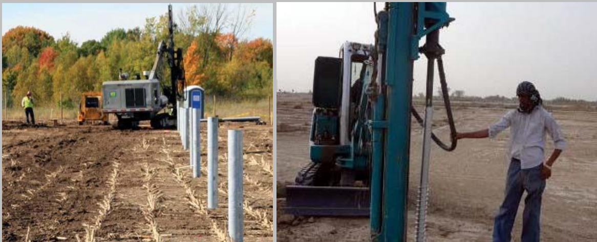
Figure 4: Driven/ Rammed Steel Pile (left) and Ground Screw (right) are the preferred mounting technology (PV Magazine, 2019)
