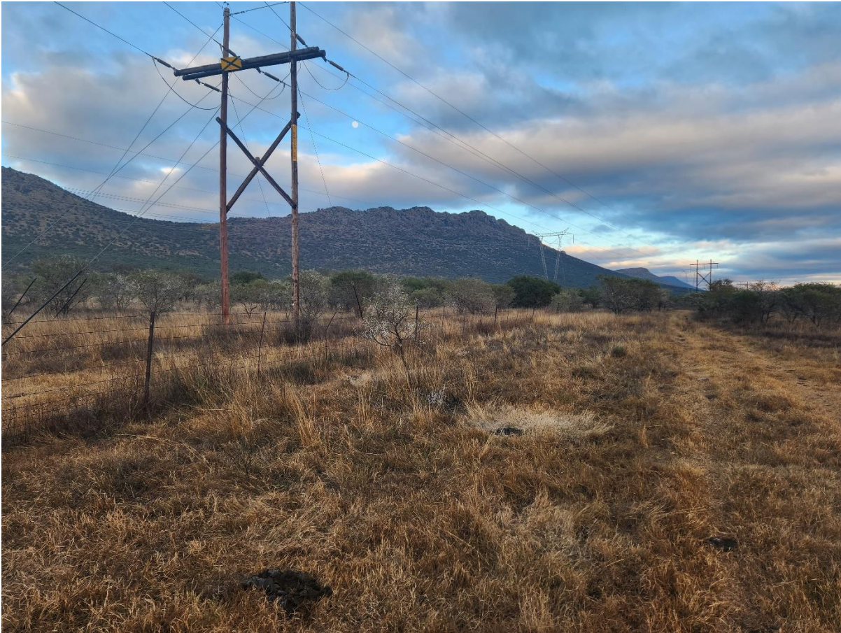
Figure 7: Existing Eskom 132kV Powerline. The proposed project will loop in and out of this powerline.
