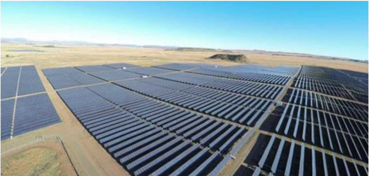
Figure 2: Aerial view of PV arrays (Photo: Scatec South Africa)
