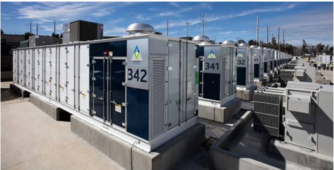
Figure 4: Close up view of a BESS (Photo: Greenbiz.com)
