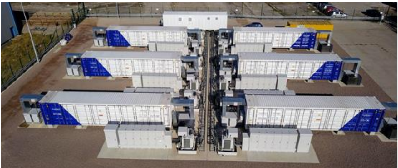
Figure 3: Aerial view of a BESS (Photo: Power Engineering International)
