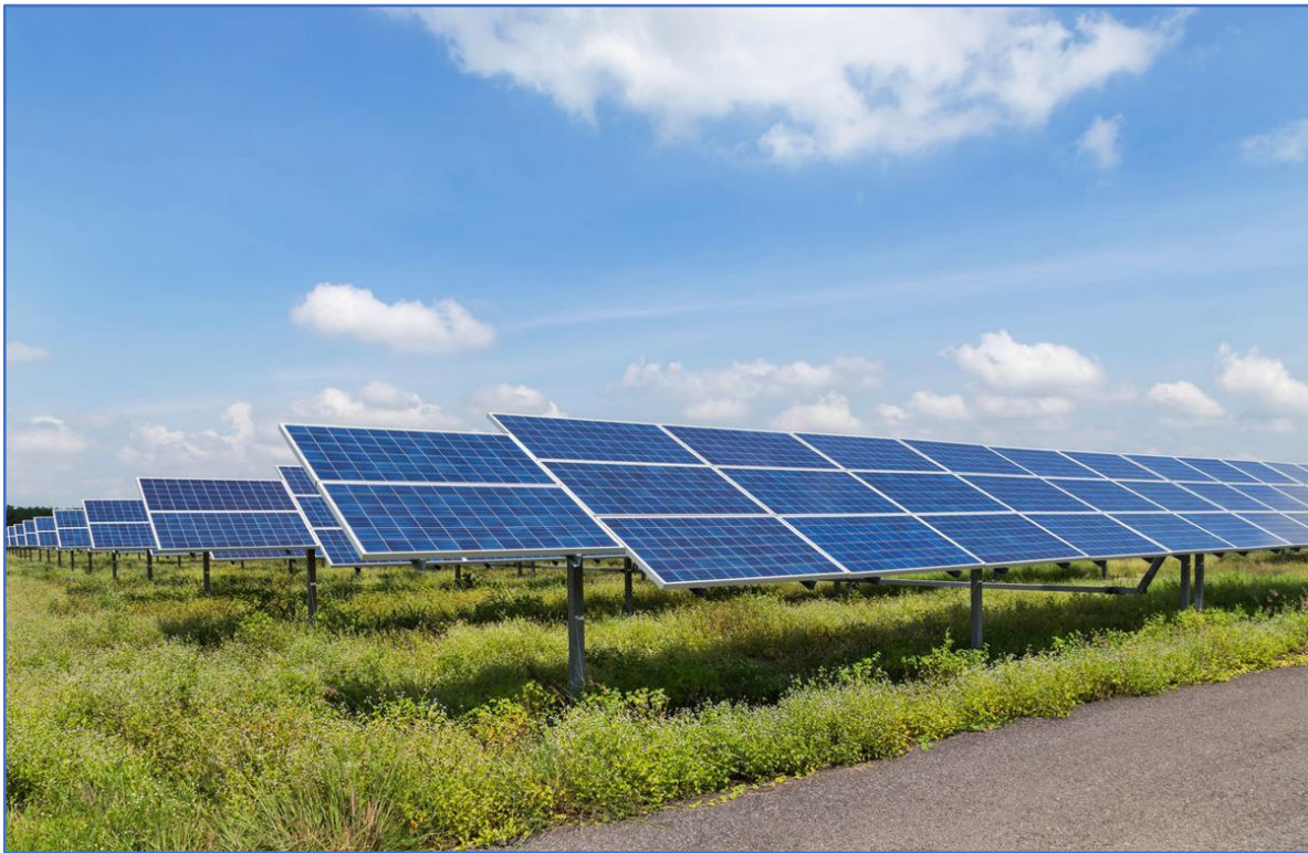
Photograph 1.1: Typical PV SEF facility
