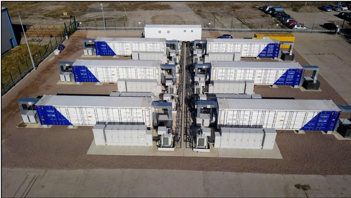
Photograph 1.2: Example of BESS located in storage containers
