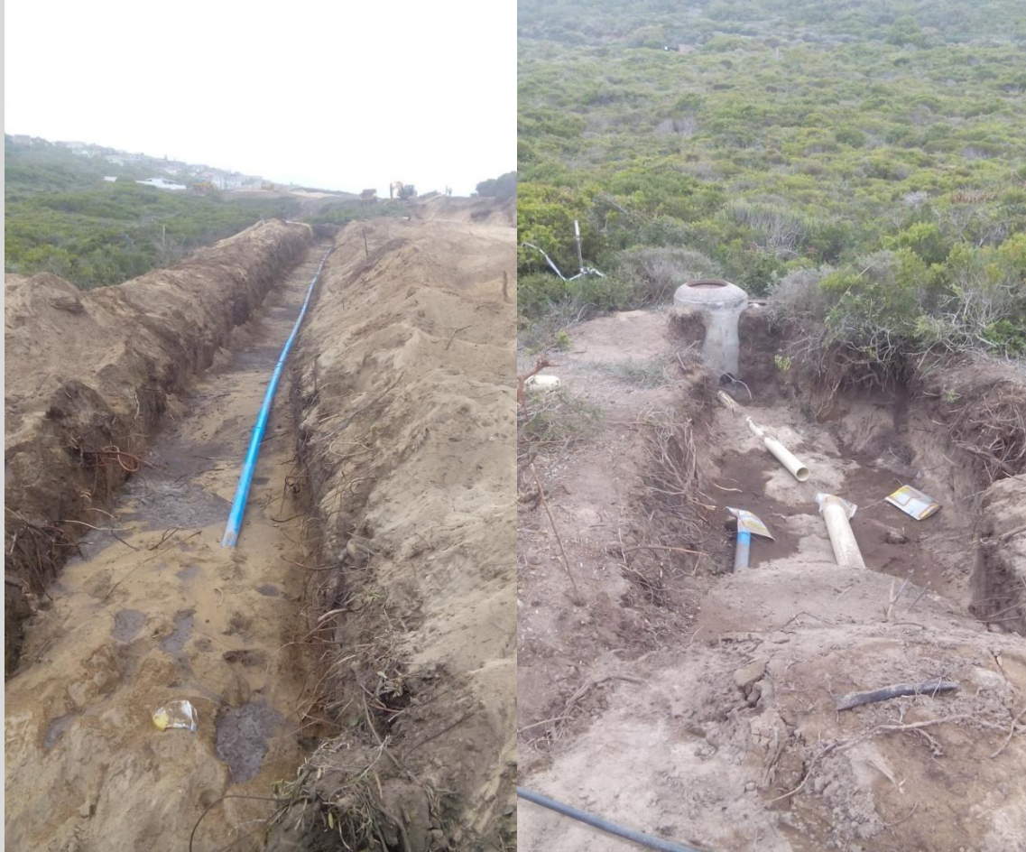
Figure 2: The bulk sewer line for the development and the connection to the existing municipal sewer outfall was completed.
