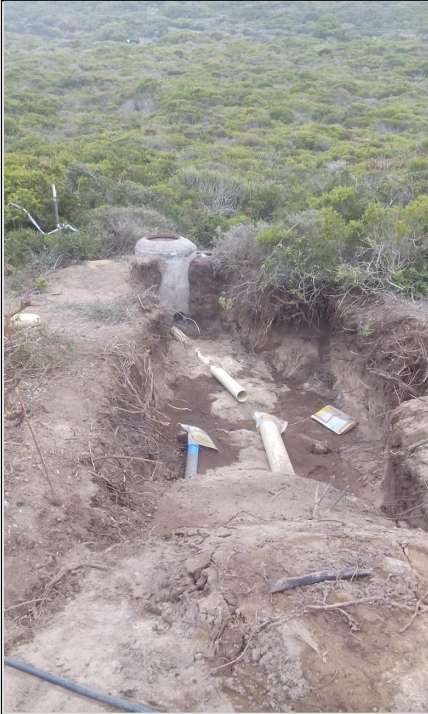
Figure 6: Installation of the bulk sewer pipe and connection the bulk municipal sewer outfall on site.
