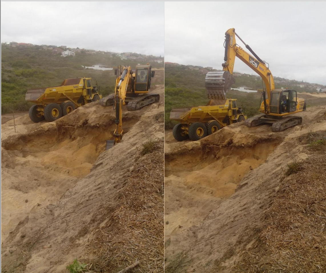
Figure 9: Showing construction of the Box Cut for the access road situated North of the Building platform.
