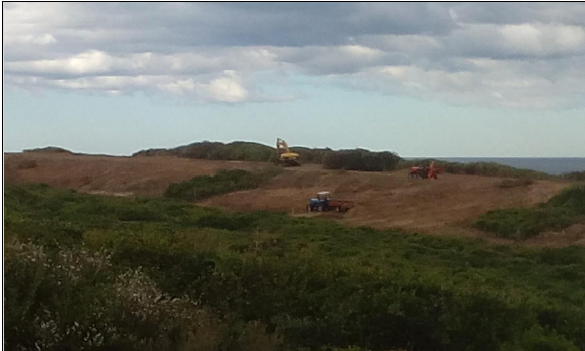
Figure 10: Showing the clearing and de-stumping of the site. The total authorised development footprint has been cleared and de-stumped.
