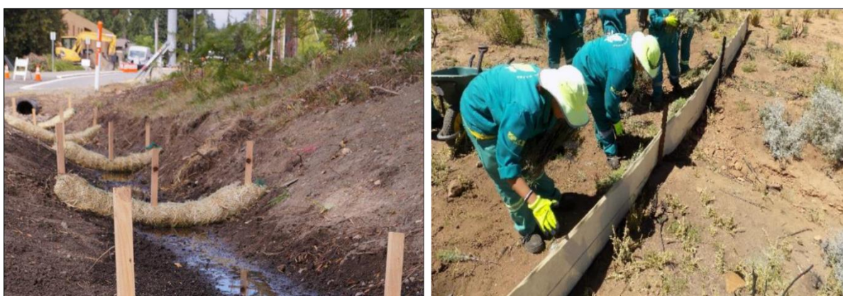
Figure 17. Examples of silt socks (left) and a silt fence (right) placed perpendicular to the flow of water. These methods reduce the force of water flow, erosion and can prevent unwanted sedimentation a site.
