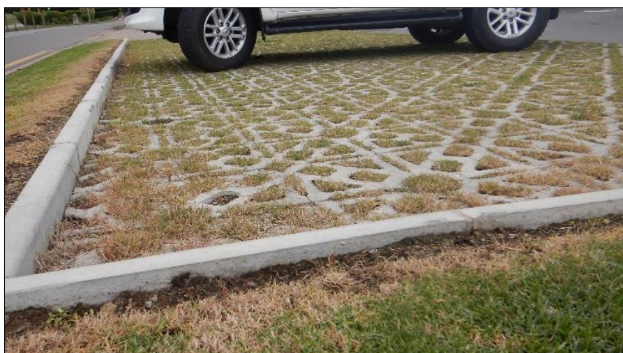
Figure 15. Examples of open pavers to use for parking areas, access roads or underneath gutters/water tank overflow areas to improve water infiltration and prevent soil erosion.
