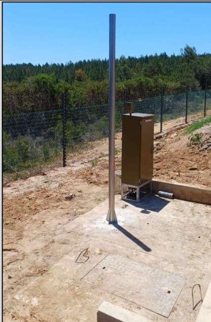
Figure 22: Typical pump station configuration, viewed from above natural ground level (NGL), showing manhole covers, a control panel and a vent pipe.
