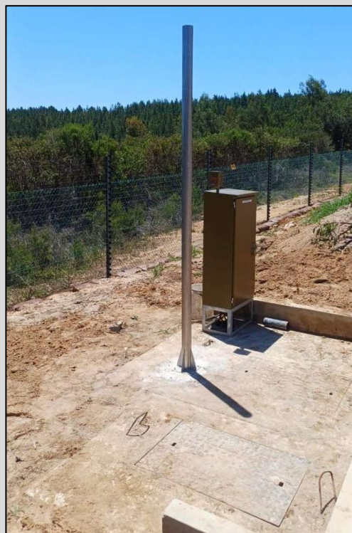
Figure 4: Typical pump station configuration, viewed from above natural ground level (NGL), showing manhole covers, a control panel and a vent pipe.
