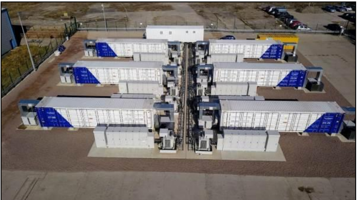
Photograph 1.2: Example of BESS located in storage containers
