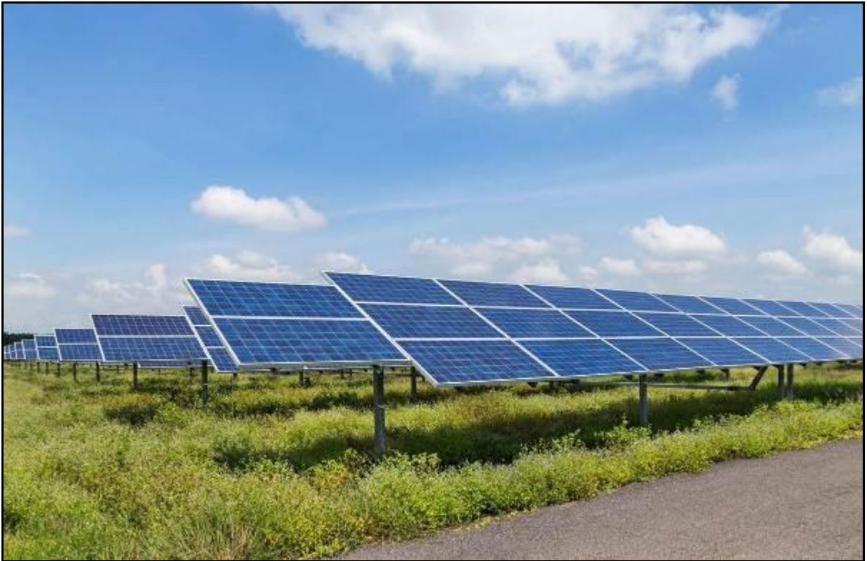
Photograph 1.1: Typical PV SEF facility
