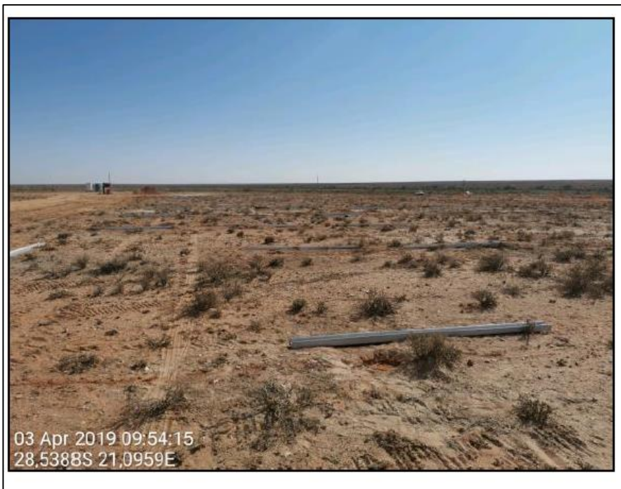
Figure 7: pre-drilled holes are backfilled with a wet sand mixture and steel piles placed in position ready for ramming.
