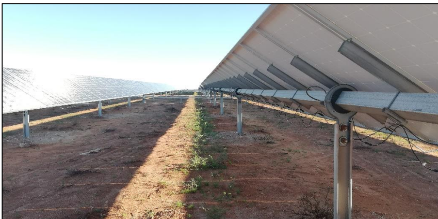
Figure 10: Showing vegetation re-establishing along the driplines of the arrays within weeks after installation.
