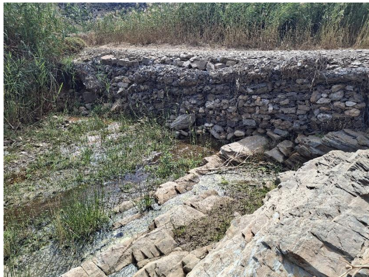
Figure 4. Photo of the existing road crossing the Jan Rolms River on gabions.
