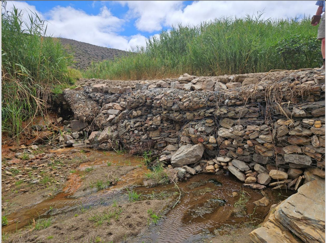
Figure 10: Existing gabion structure that forms the access over the Jan Rolms River which forms an obstruction in the riverbed to be replaced with box culverts that will improve hydrology.
