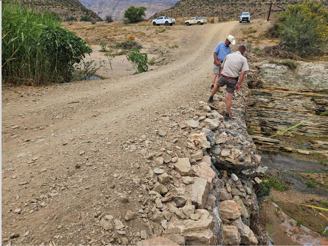
Figure 8: Section of the existing crossing over the Jan Rolms River with gabions obstructing flow.
