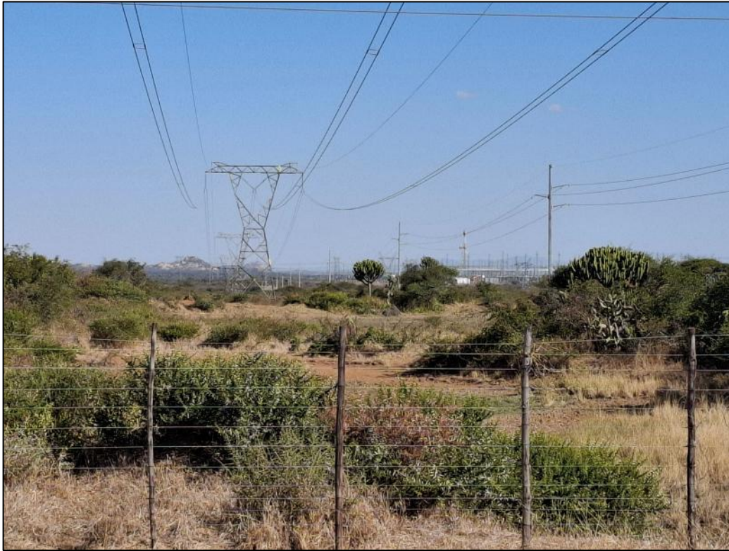
Photograph 3.8: Eskom transmission lines entering Tabor Substation
