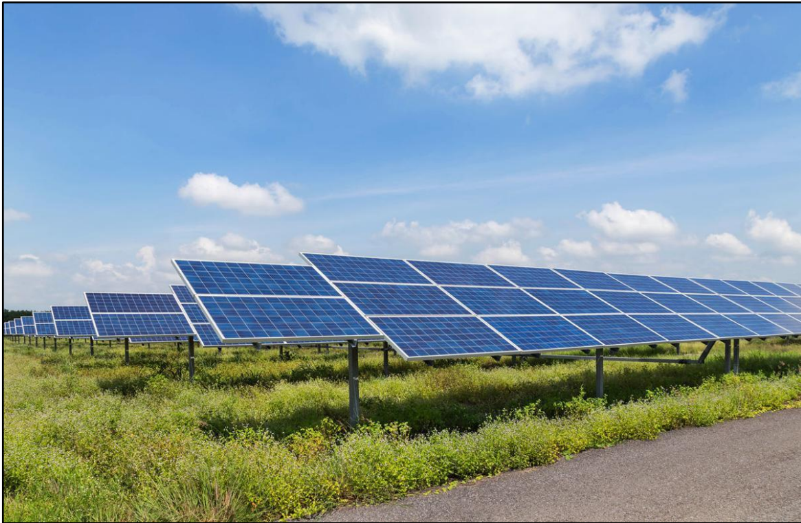
Photograph 1.1: Typical PV SEF facility
