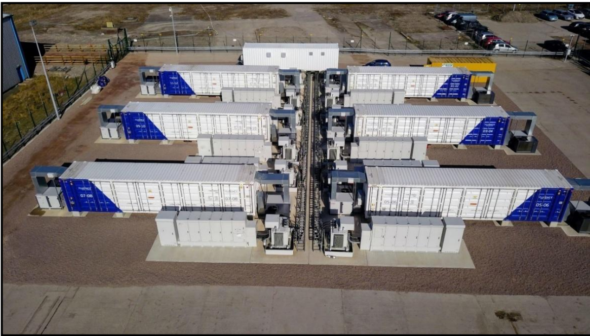
Photograph 1.2: Example of BESS located in storage containers
