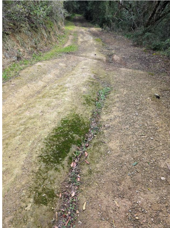
Erosion gulleys forming in surface or road due to insufficient drainage and stormwater management because side drains are no longer functional.
