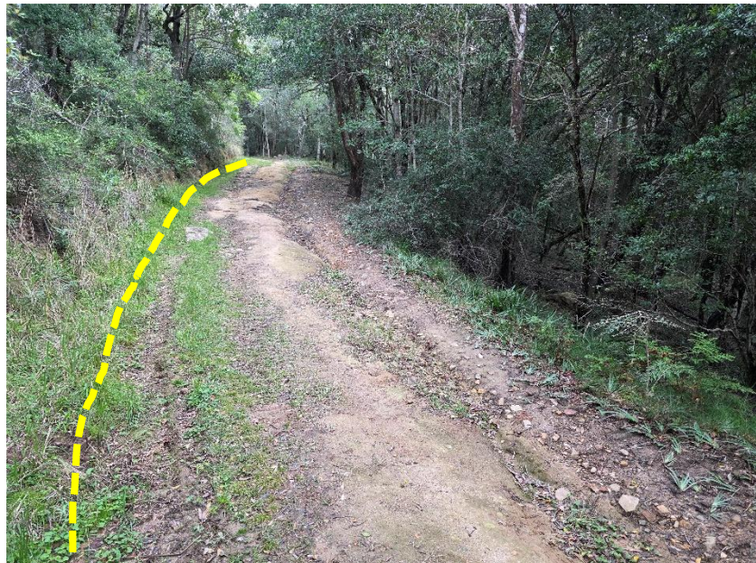
Existing side drain along the road is silted up and blocked, therefore stormwater runs over and into the road resulting in erosion. Side drains must be opened/vegetation regrowth cleared to be functional and stone pitching recommended to improve sustainability.
