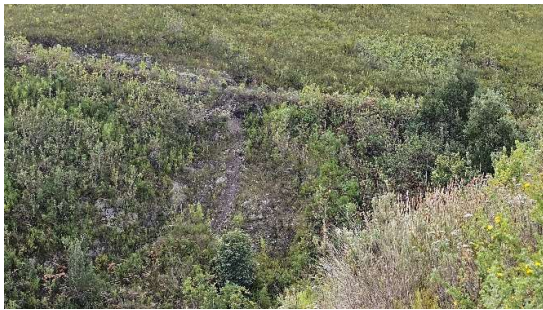
Figure 15: Photo 11, signs of slope failure or slip observed from a photo taken from a distant vantage point.
