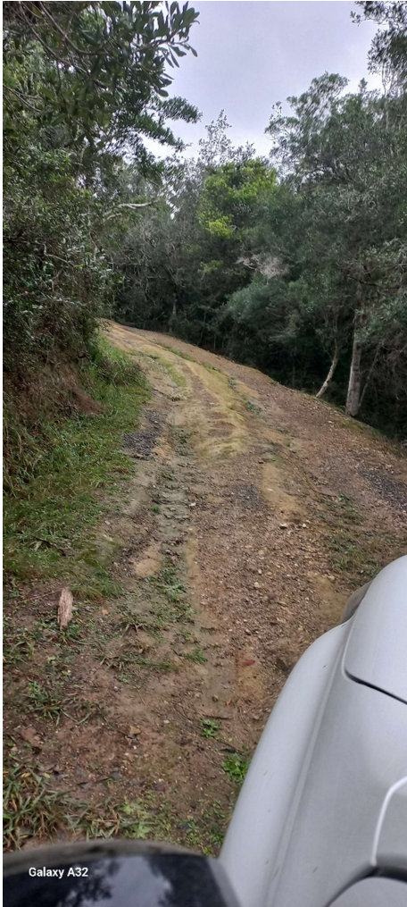
Figure 18: Photo 6, road is in poor condition, with significant rutting and muddy wheel tracks.
