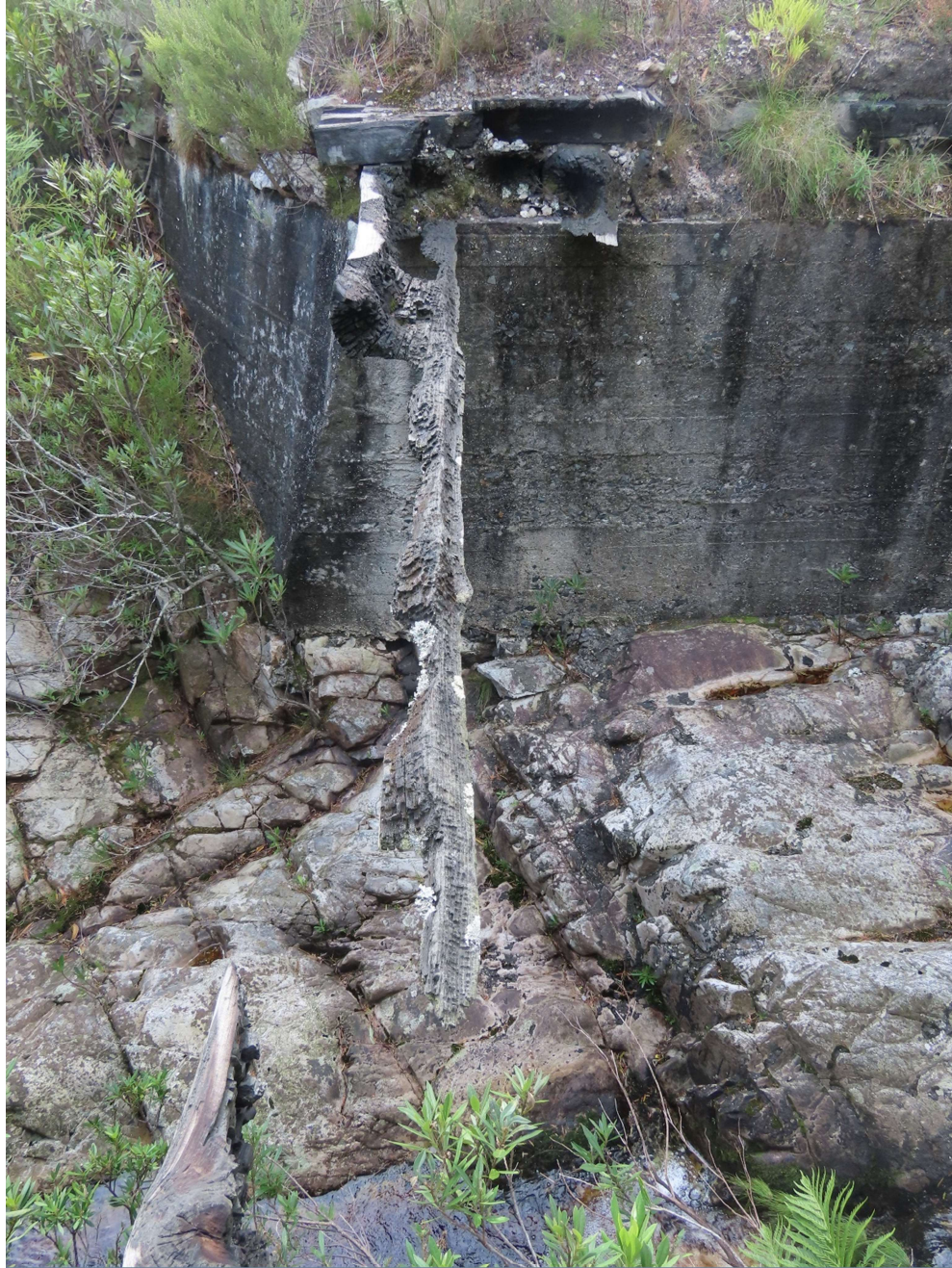
Figure 8: Photo 5, remnant of burned wooden bridge deck.
