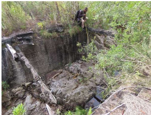
Figure 17: Photo 20, burned-down bridge.
